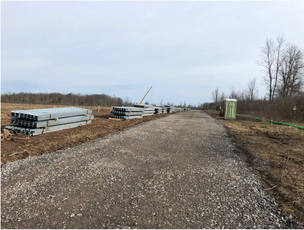
The view of a planned, 7-megawatt solar array under construction on Whitehaven Road. Crews soon will drive these metal piles into the ground. (Stephen T. Watson/Buffalo News)
