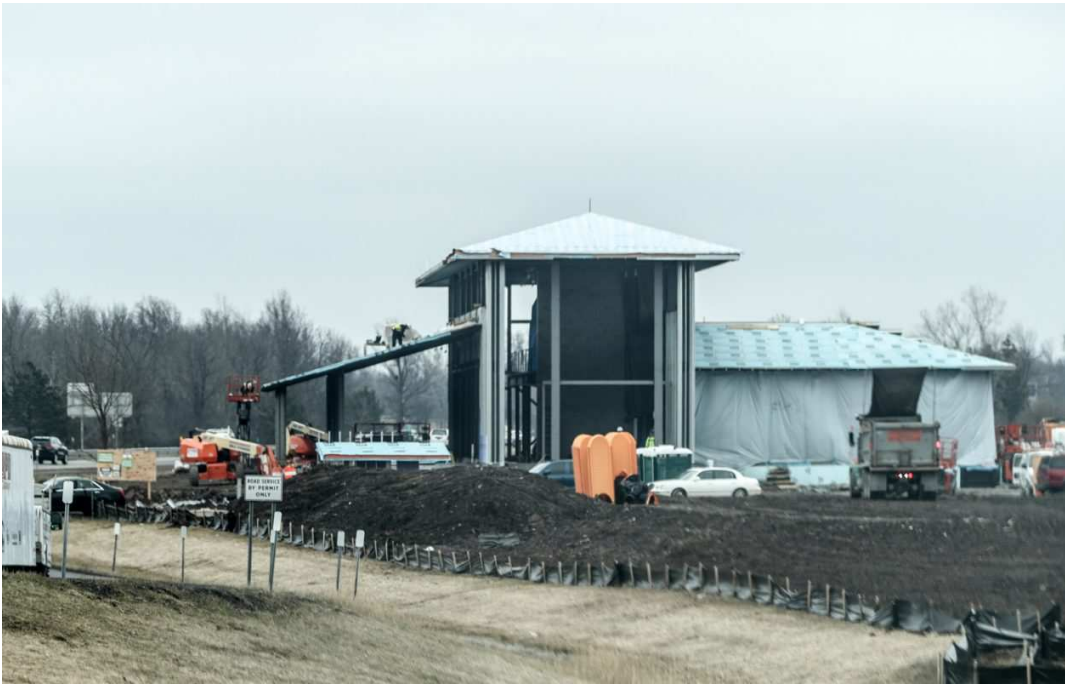
Photos of construction work in progress at the Grand Island Welcome Center. (James P. McCoy/Buffalo News)
